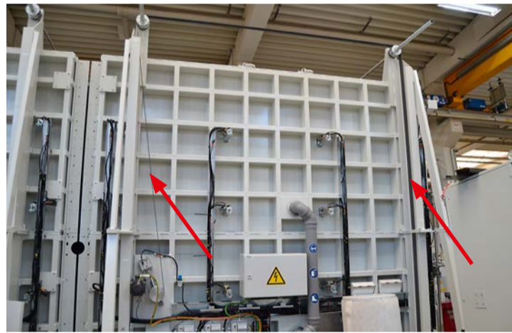
View from the rear of one of the five assembly and gas filling presses installed side-by-side.
